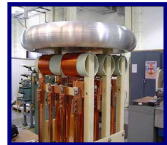
SuperPower's FCL module testing
